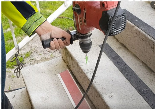
Using the countersunk holes as a guide, drill a much larger hole to accommodate a plug.
