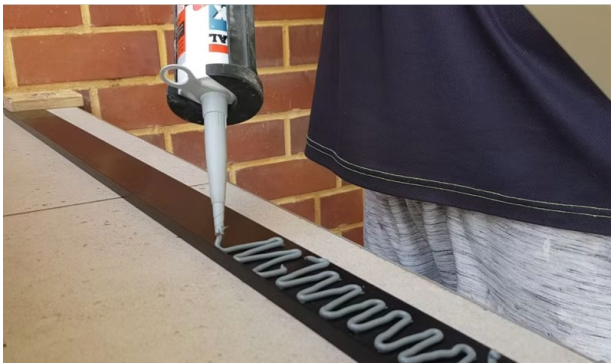
Using a caulking gun, apply Soudal adhesive in a snake like fashion to the back of the nosing.
